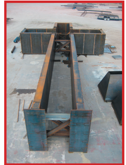
The massive cross is ready to be delivered to Kerrville from Wyoming.
